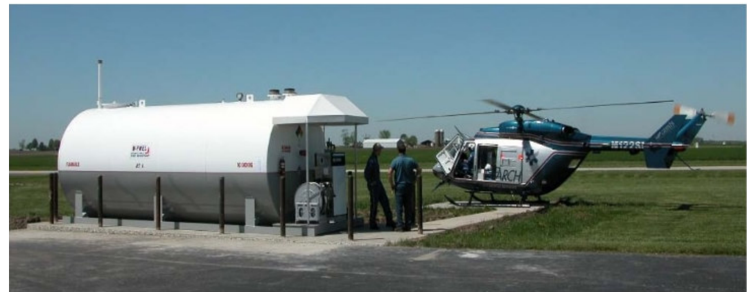
Complete unitized fueling facility, MSi
